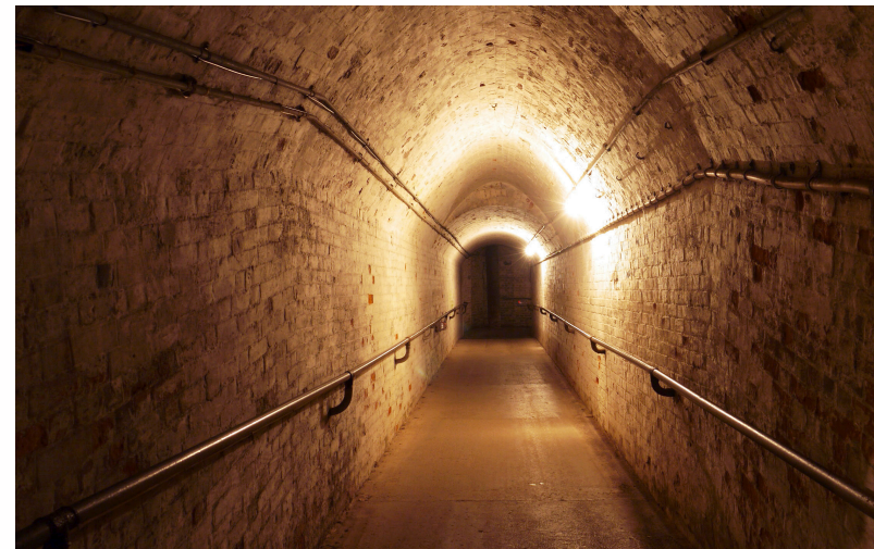
1c Existing and replacement bell jar luminaires illuminate the vaulted corridors. Lamp type: A1
